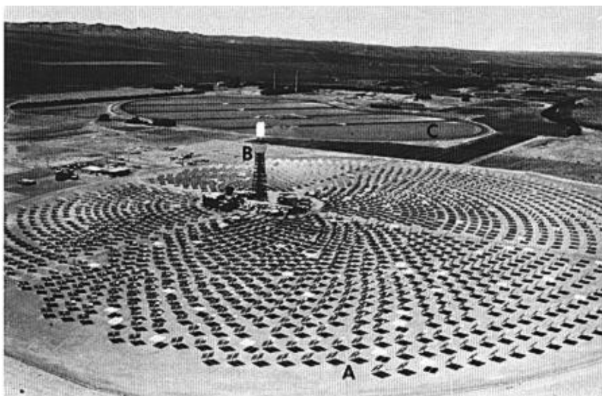
FIGURE 1. Aerial view of Solar One: (A) heliostat field, (B) central receiver tower, (C) evaporation ponds. Tower height = 86 m, diameter of field = 765 m.
