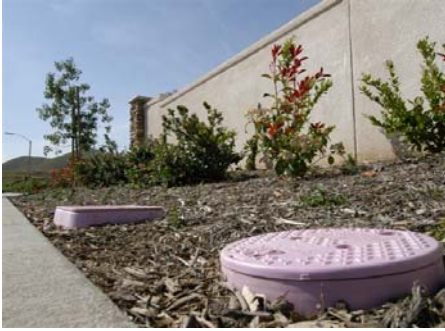
Photo Credit: Eastern Municipal Water District.
